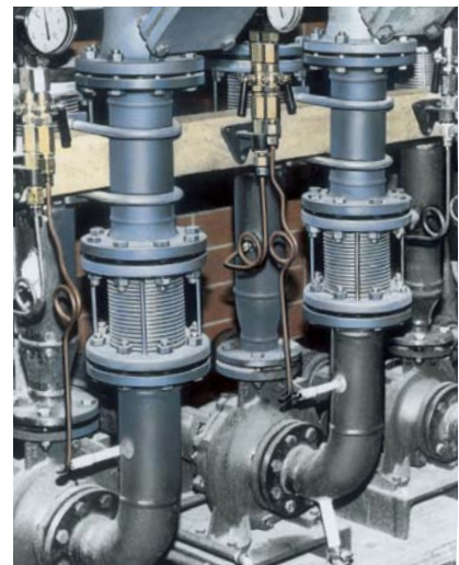
STENFLEX® type SR-2 at pumps
