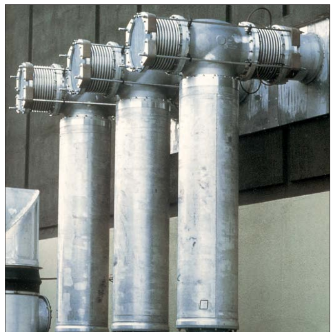
Restrained STENFLEX® stainless steel expansion joints type SF-25 to absorb thermal expansion in a transformer plant
