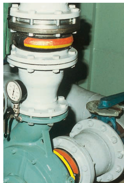
STENFLEX® type AR-1 used at pumps
