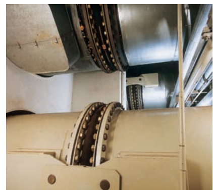
STENFLEX® type C-1 with special high restraints in cooling water system of a power plant
