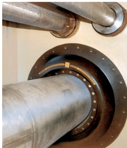
STENFLEX® type W-2 in a power plant
