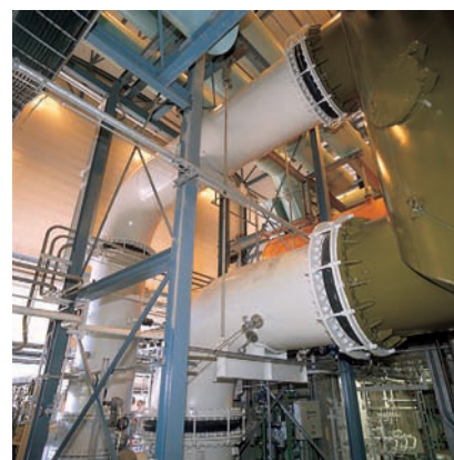
STENFLEX® type C-31 in a power plant
